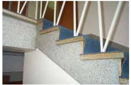
Figure C5: Detail of the stairs. Note the terrazzo stringer and treads, as well as the wrought iron balustrade. OCP 2006
