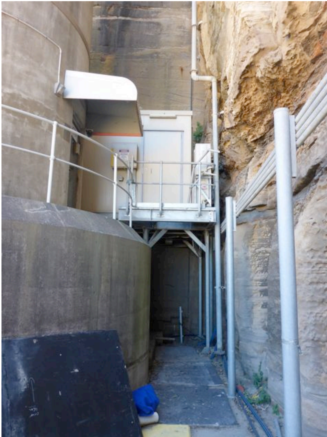
Figure 4.4. Base of HCT viewed to north. Note the large base plinth with walkway and handrail and entrance door at left, the cliff face at right and rear, and a small external (plant?) room with two split system airconditioning units on its right. (Photo Austral Archaeology Pty Ltd, October 2013)
