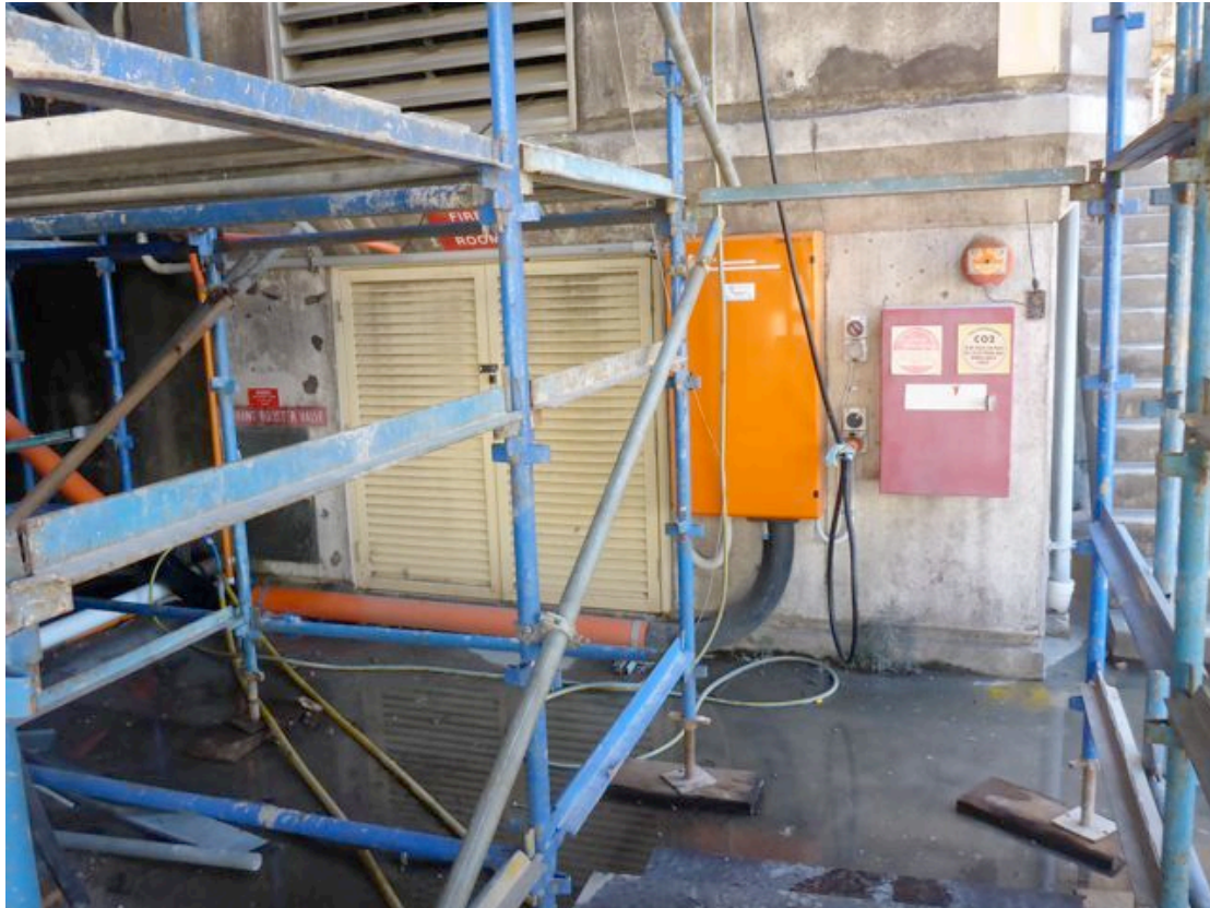
Figure 4.5. Base of HCT viewed to the east. Note the lower louvred doors provide access to the Fire Room and the upper louvred vent provides ventilation to the western end of the Switch Room. (Photo Austral Archaeology Pty Ltd, October 2013)
