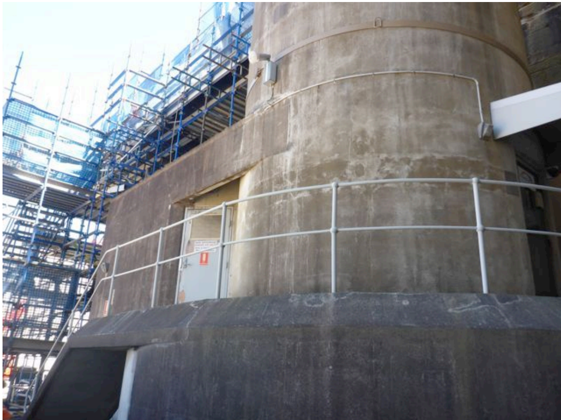
Figure 4.2. Base of HCT viewed to northwest. Note the large base plinth with walkway and handrail above and main switch room door visible at left and lower main entrance door at right. (Photo Austral Archaeology Pty Ltd, October 2013)
