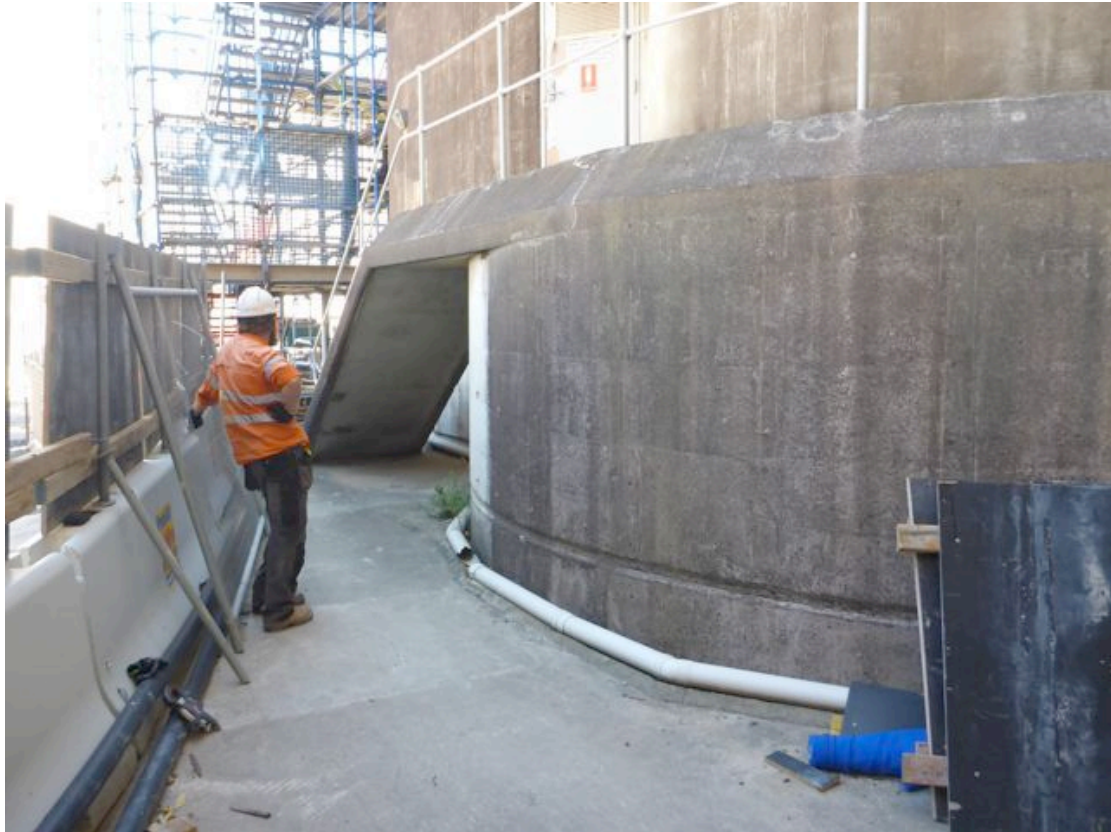
Figure 4.3. Base of HCT viewed to west. Note the access stairway to the walkway on the large base plinth. (Photo Austral Archaeology Pty Ltd, October 2013)
