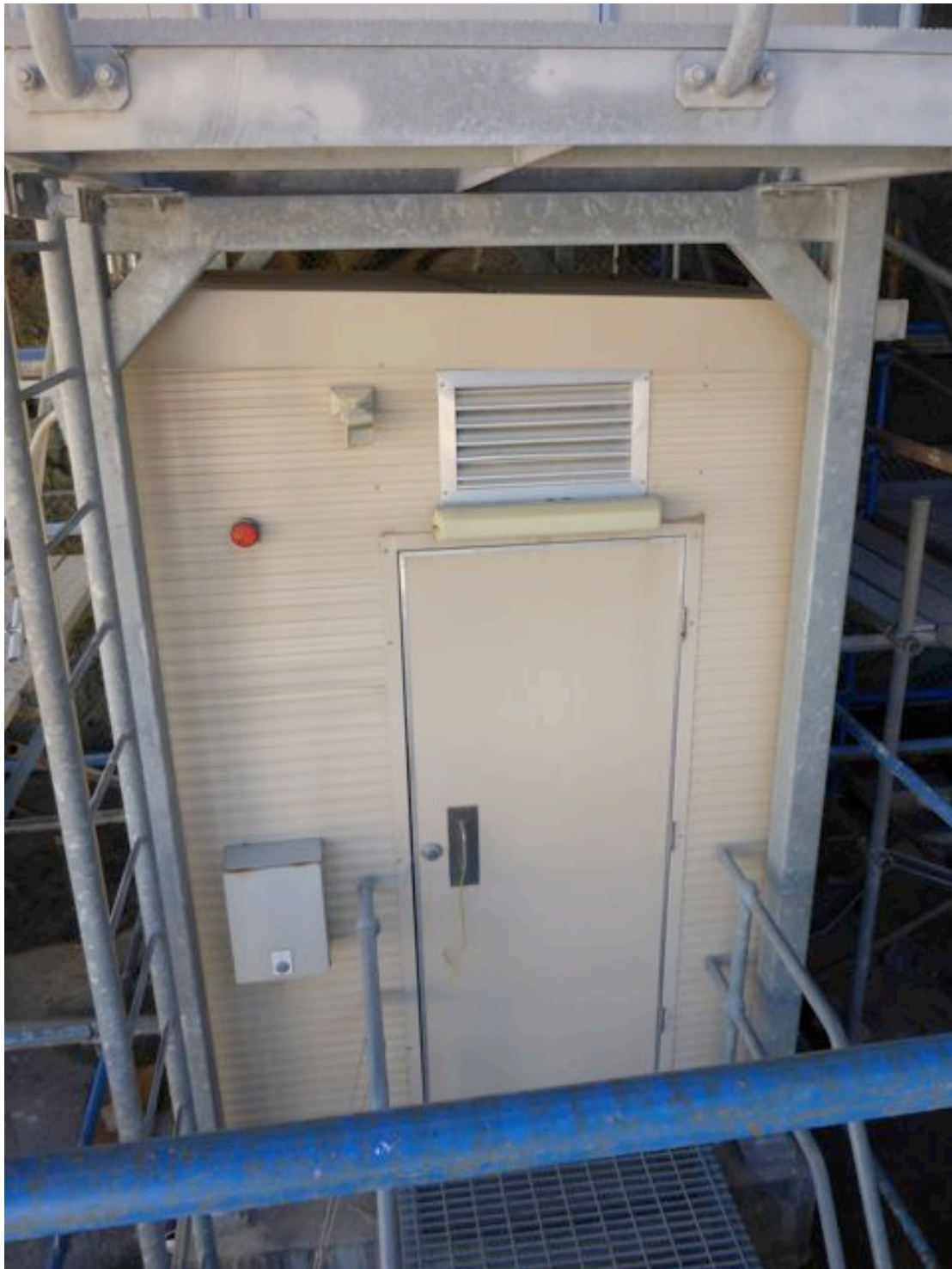
Figure 4.6. View to the north of the lower level of the freestanding Telstra plant room located on the west side of the tower base. (Photo Austral Archaeology Pty Ltd, October 2013)
