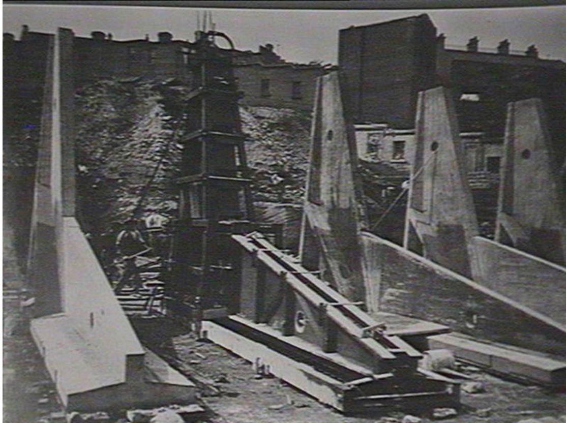
Reinforced concrete trestle used for retaining and sea walls in construction at Millers Point (Government Printers Office image City of Sydney archives).
