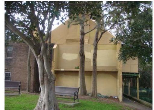
Fig. 3.8: Western wall of Munn Street Terraces with evidence of adjoining building since demolished.
