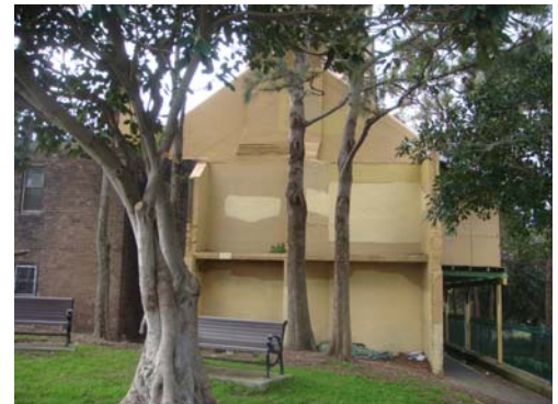
Fig. 3.8: Western wall of Munn Street Terraces with evidence of adjoining building since demolished.
