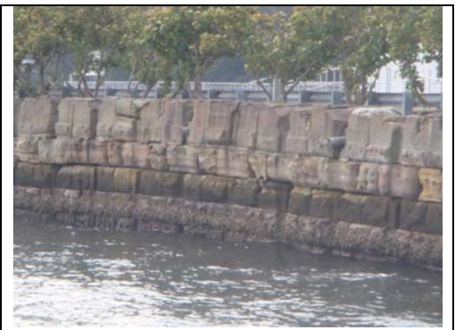
Fig. 3.4: Sandstone seawall with existing site stormwater pipes penetrating through.
