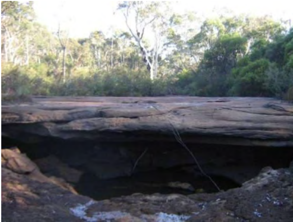
Photograph 4.3 Creek bed collapse in Lizard Creek
