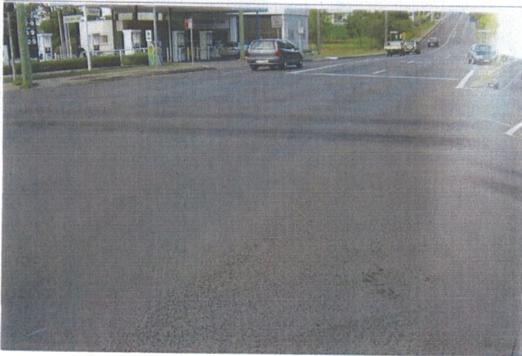
Road runs black after one day of road haulage October 2010. This happens all the time. This is excessive dust deposits on the road. (Exit from NRE mine onto Bellambi Lane)
