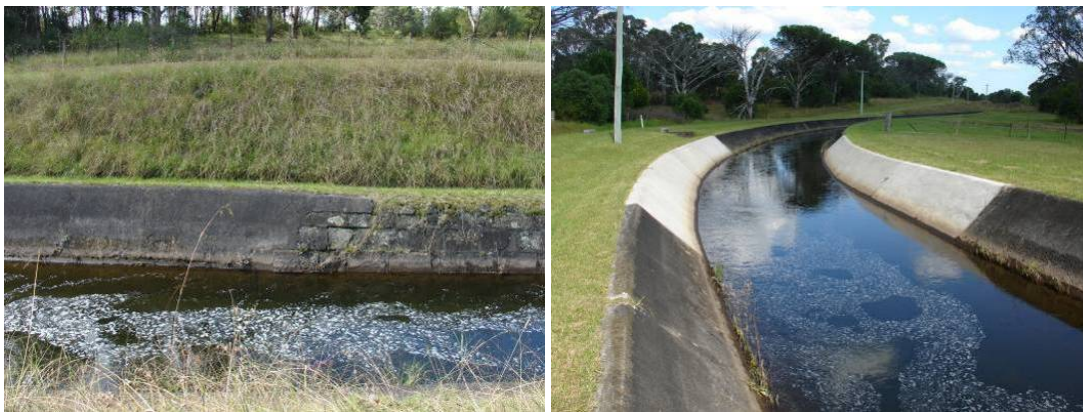
Figure 5.29 View to the east sandstone block wall with concrete lining (left) and view of a new concrete section.
