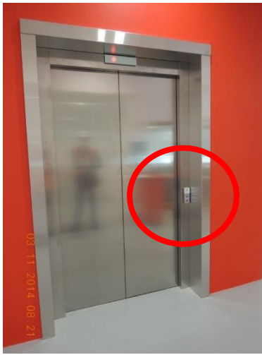
Figure 2 image of non-compliant lift call button installation
