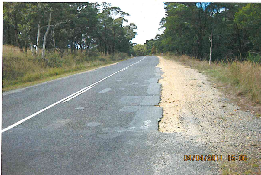
Figure 15: Damaged shoulder of Bungendore Road (Palerang Council, 2011)
