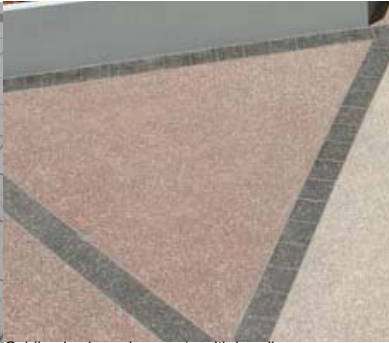
Oxidised coloured concrete with banding.
