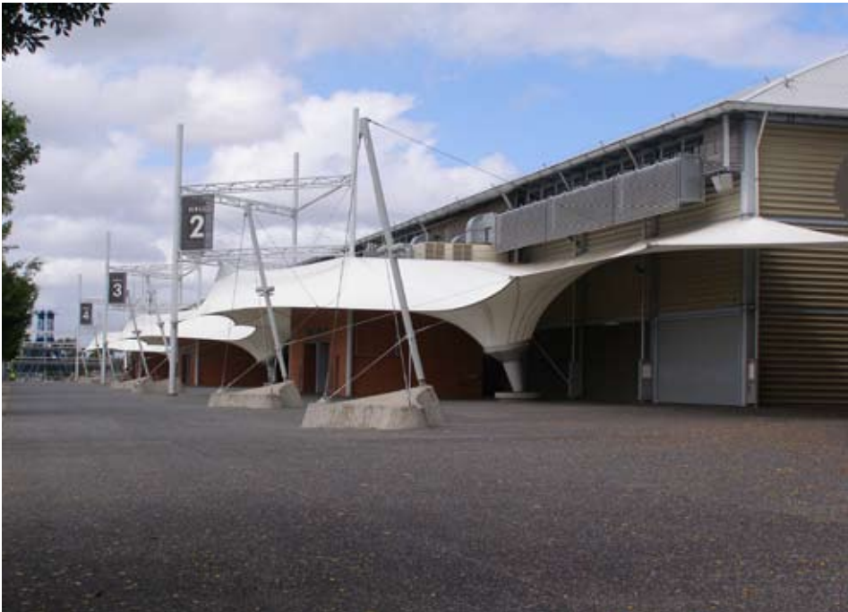
Figure 7 – Existing entrances and service pods on the northern elevation of the hall
