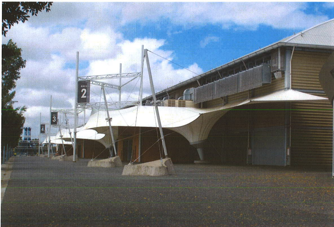
Figure 5 – Existing entrances and service pods on the northern elevation of the hall
