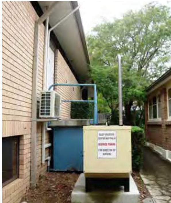
Photo 13: Power system connecting to southern side of San Day Surgery building
