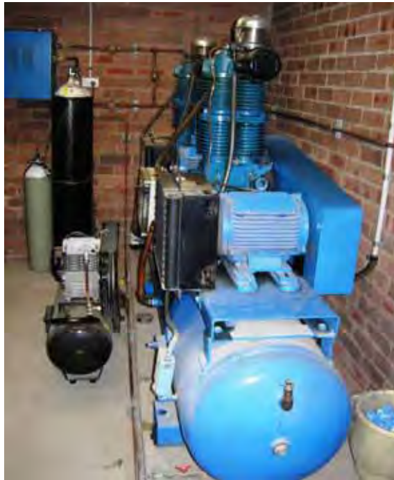
Photo 18: Compressor inside non-flammable gas store room within Surgery basement
