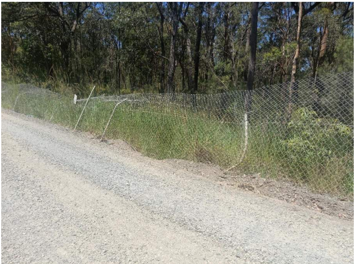
Plate 13: Damaged fence along western boundary of haul road
