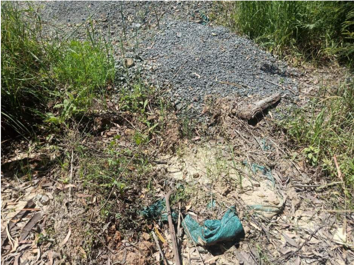
Photo 1 Sediment fencing down and overtopping within Lot 12.
