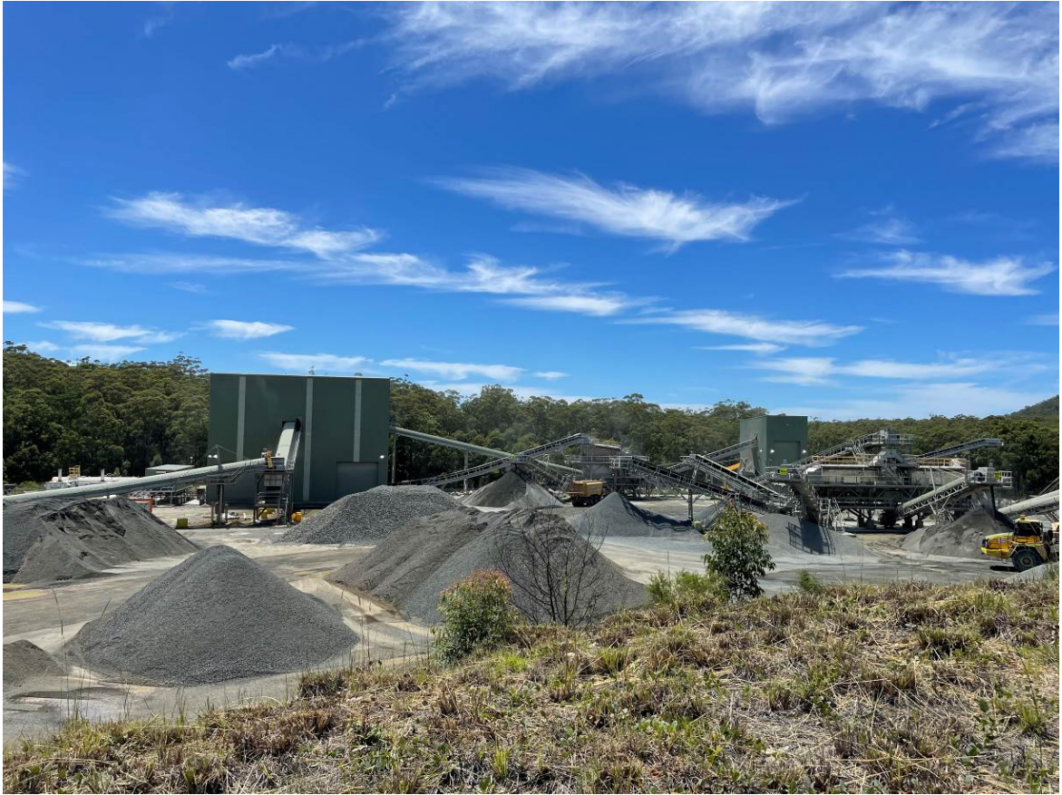
Photo 1 –Crushing Plant (January 2021)
