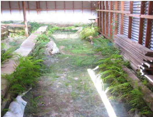
Most noticeably prevalent along the northern side of the Convict Hut
