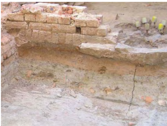
Erosion has caused an undercut of a brick wall on the south side of the site
