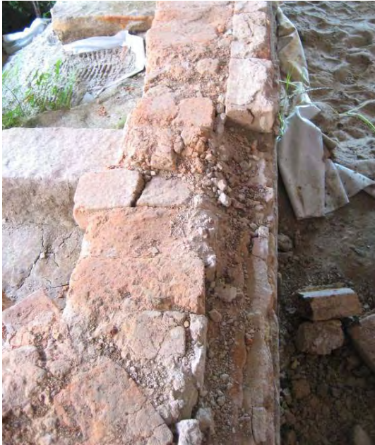
Evident along most brick wall features.
