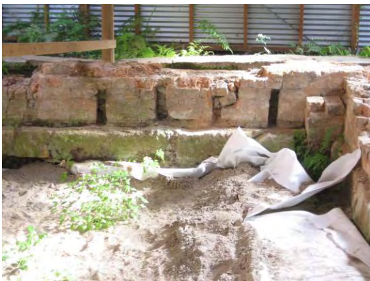
Also evident on the lower courses of brick / stonework of the northern walls.
