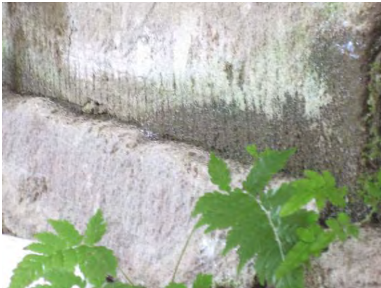
Efflorescence evident on vertical faces on most brick and stone wall features.
