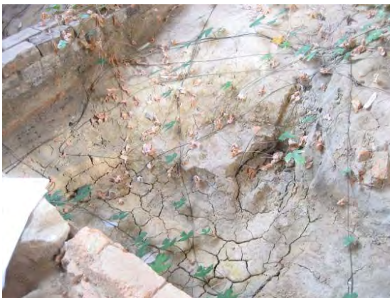
Soil cracking is evident as the ground dries out
