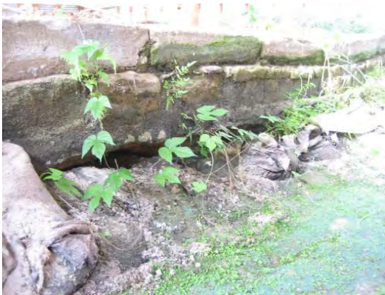
Evident along the wall on the north side of the Convict Hut
