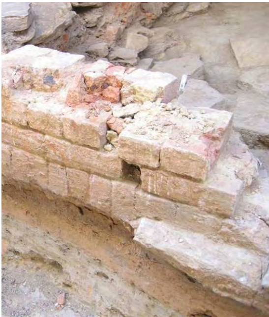
Degree of crumbling varies from large cracks through brick remnants, to very small fine particles.
