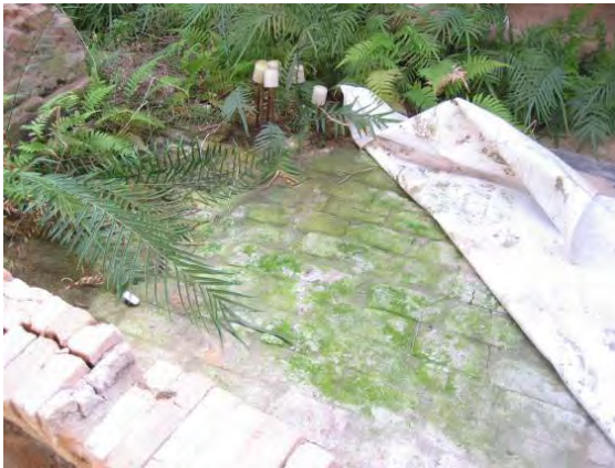
Algal growth is apparent on the horizontal feature paving in the centre of the Convict Hut remains.
