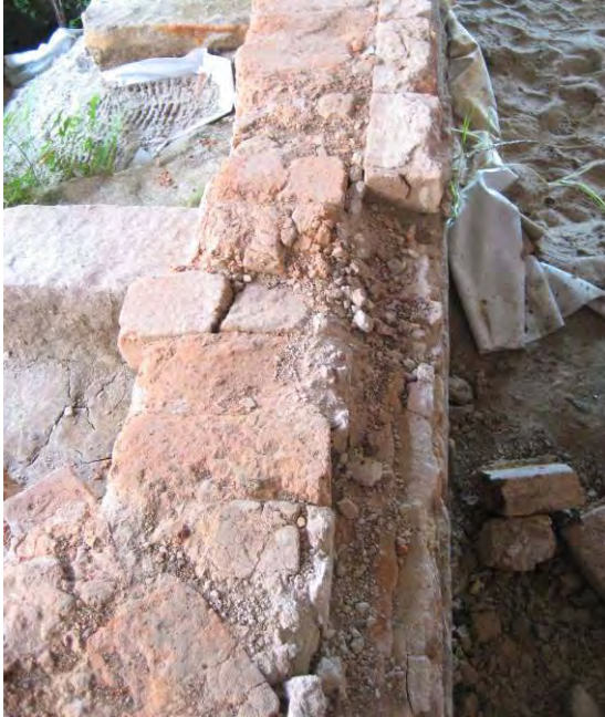
Evident along most brick wall features.
