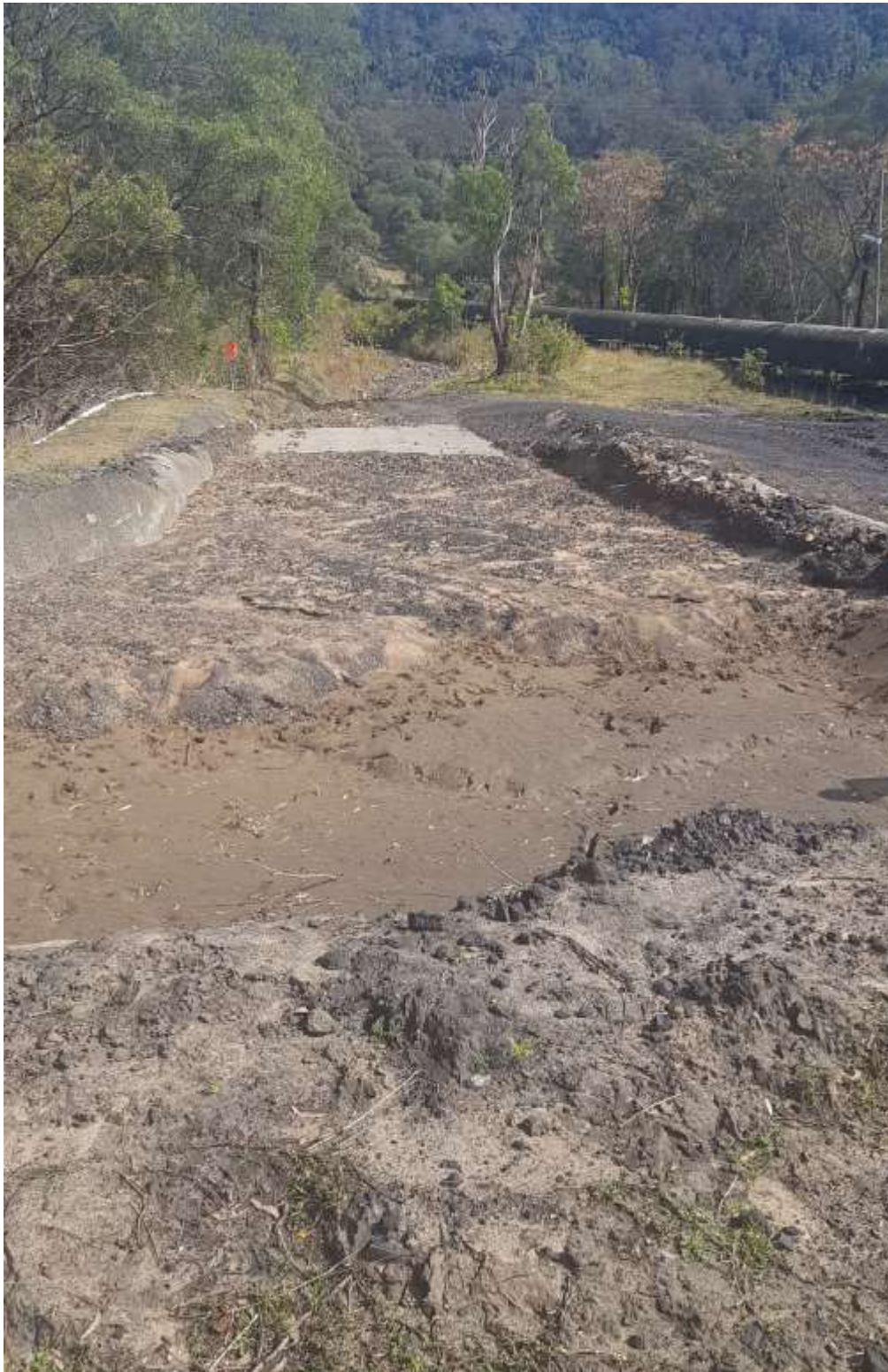
Photo 6: Catch drain with bund with evidence of overflow
