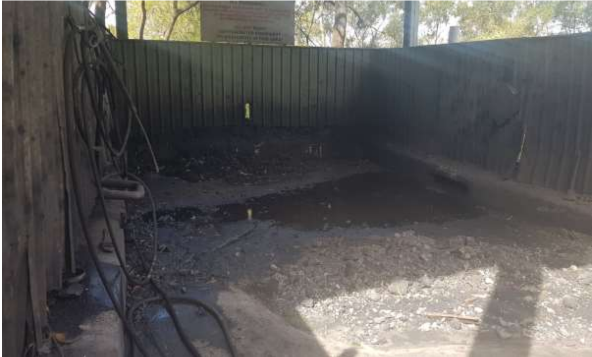
Photo 10: Wash-bay in need of maintenance
