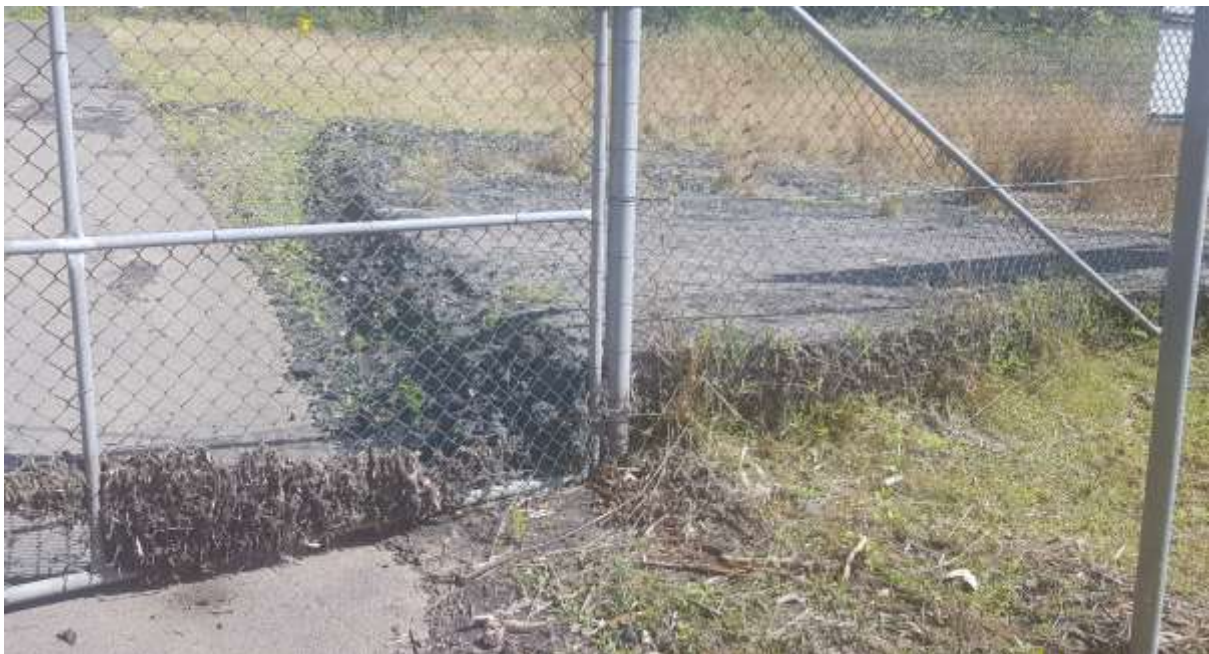
Photo 8: Example of waste coal and uncontrolled erosion.
