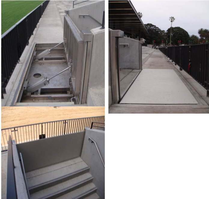
Figure 6.5 Flood Barrier – BL/HWS-K showing indicative trench depth and system in the closed and opened positions.
