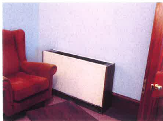
Figure 3.9 Perth House, showing floor-mounted air conditioning unit [Source: CM+, October 2004]
