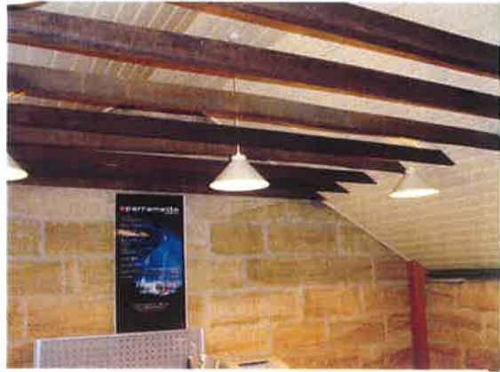
Figure 3.25 Perth House stables, Upper Floor, showing exposed rafters and roof structure [Source: CM+, October 2004]
