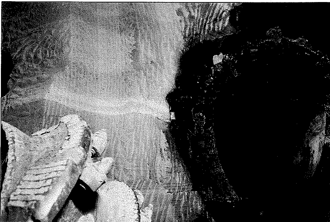
Figure 4 – Exposure of the Bennelong Drain as sliced through in the Opera House Car Park cavern.
