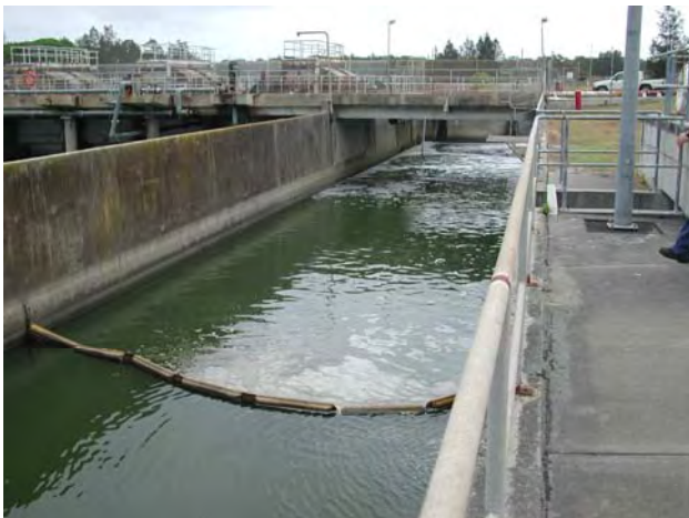
Plate 8.1 – Cooling water screens and outlet canal
