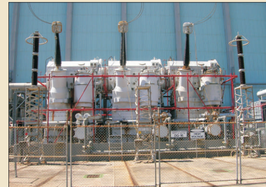
Generator transformer outside turbine hall
