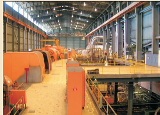
Inside turbine hall units 3 and 4
