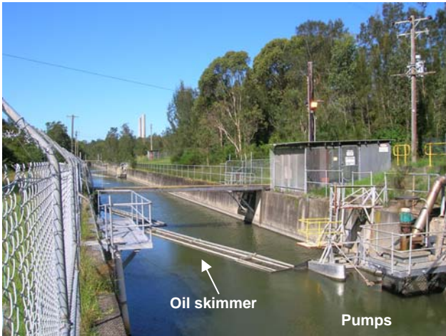
Plate 1.2 – Oil skimmer on outlet canal
