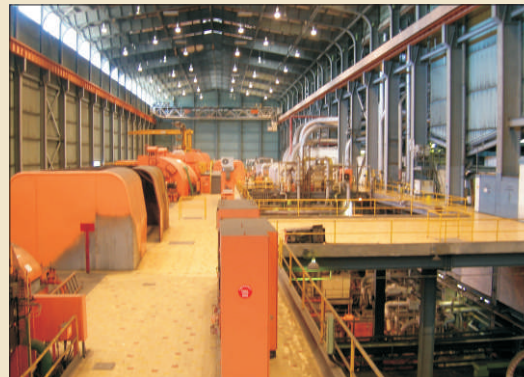
Inside turbine hall units 3 and 4
