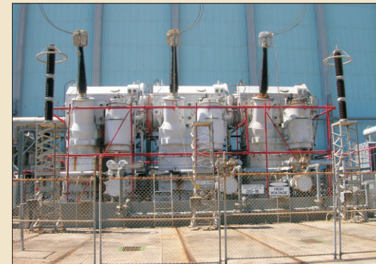
Generator transformer outside turbine hall
