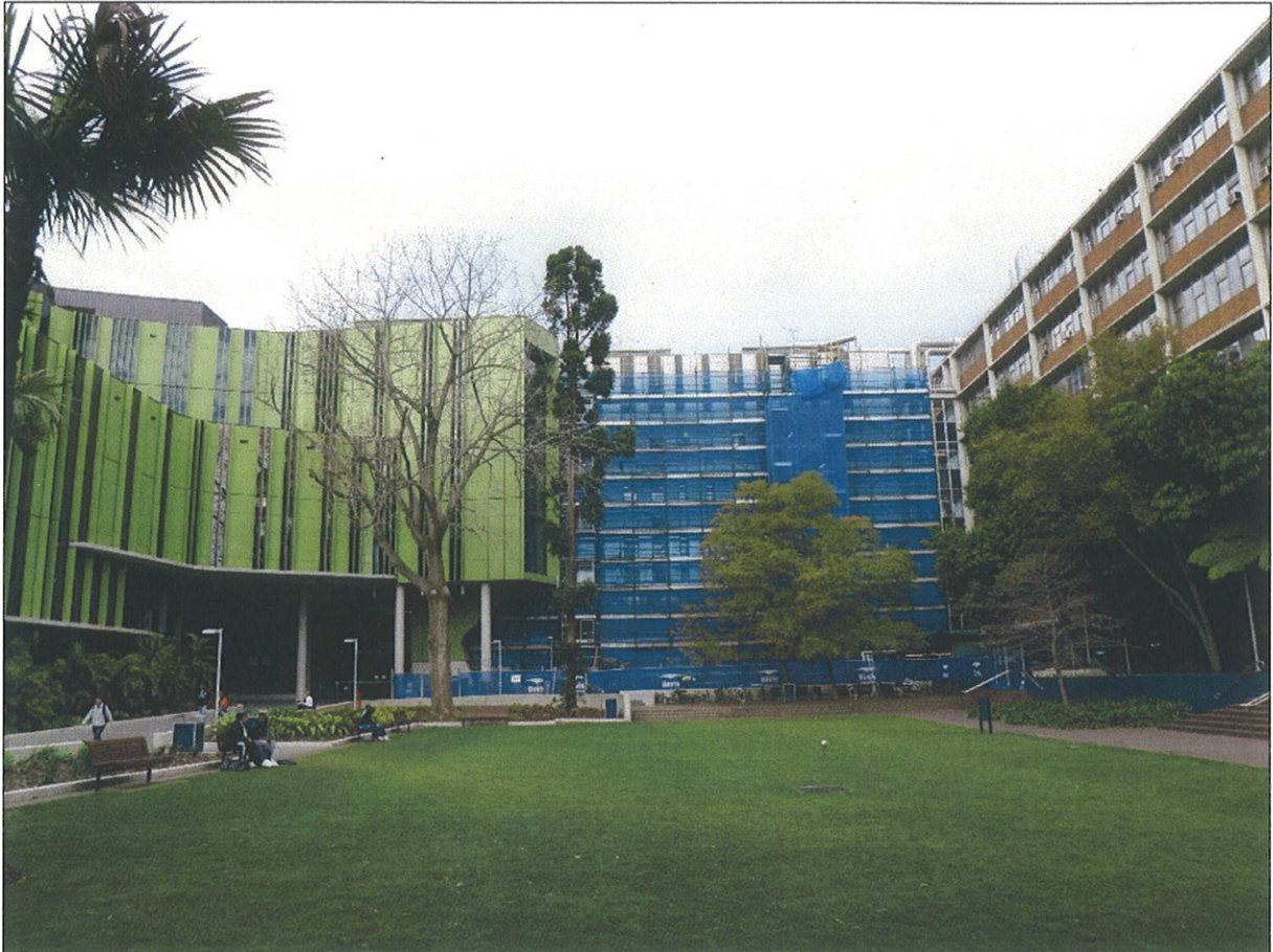
Figure 7 – View of the western elevation of existing WWB and adjacent Michael Birt Gardens, Lowy Cancer Research Building and Biological Sciences Building
