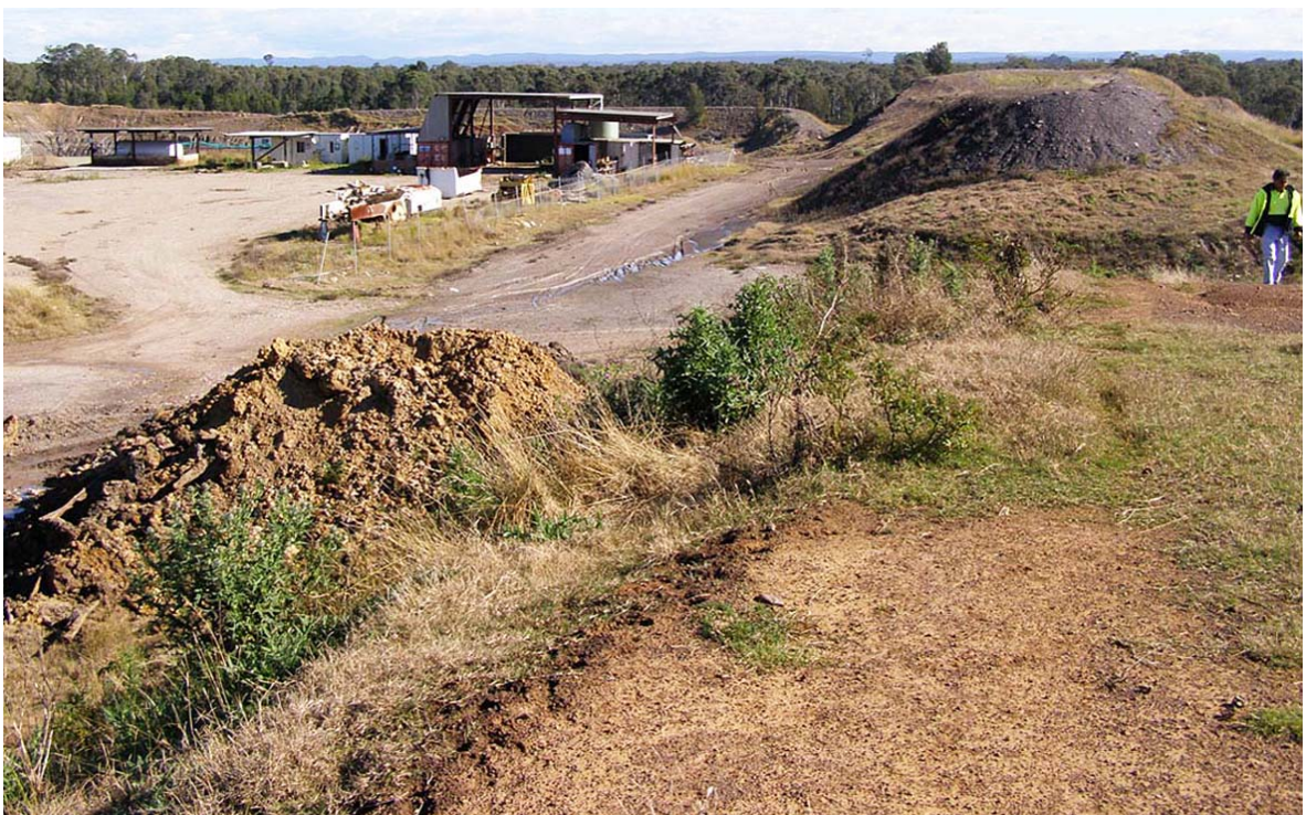
Plate 6: The equipment compound viewed from the north-eastern bundwall
