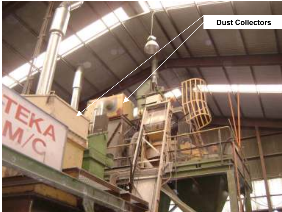
- Diagram 7 - Cookson Plibrico Bulli Plant – TEKA Machine Typical Arrangement for Dust Collectors at back end of Plant Process
