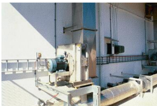
Photo C.1-5 Tunnel composting air supply system (example)
