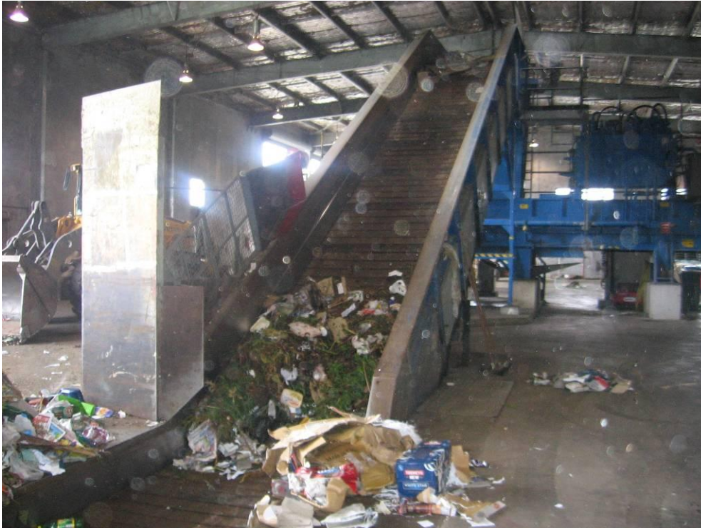
Photo B.2-8 Loading conveyor at Ballina NSW baling plant
