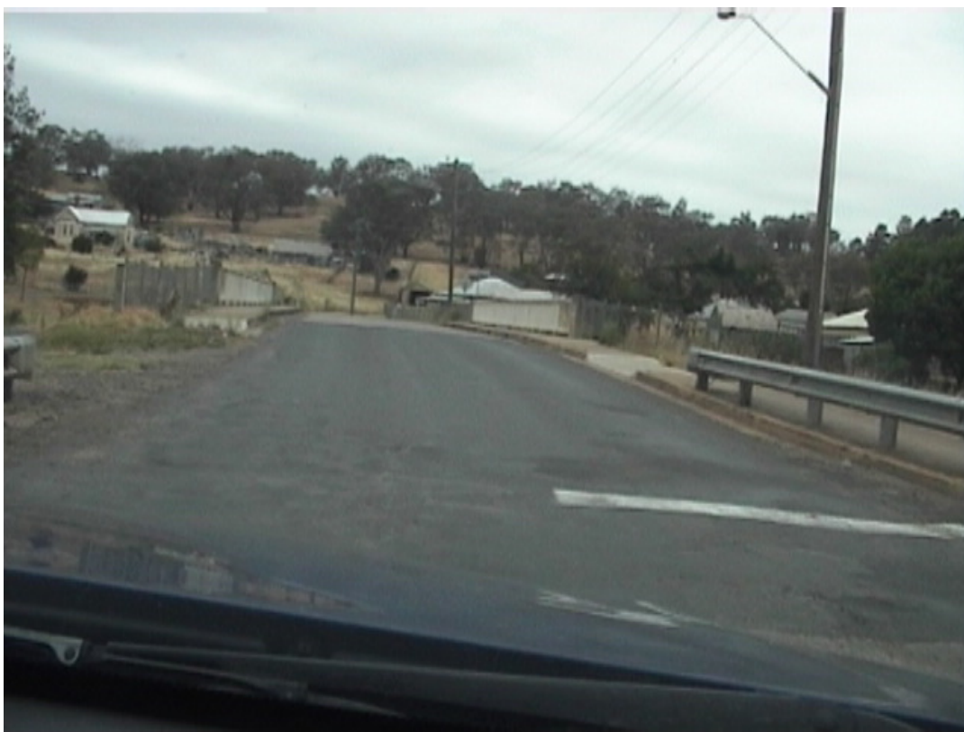
13 – Deficiency Log Item 9 In advance of the Railway Level Crossing centreline BB markings are non-existent. As the boom gates control only half of the road carriageway it is considered essential BB centreline markings be installed in accordance with AS 1742.11 Railway Level Crossings.
