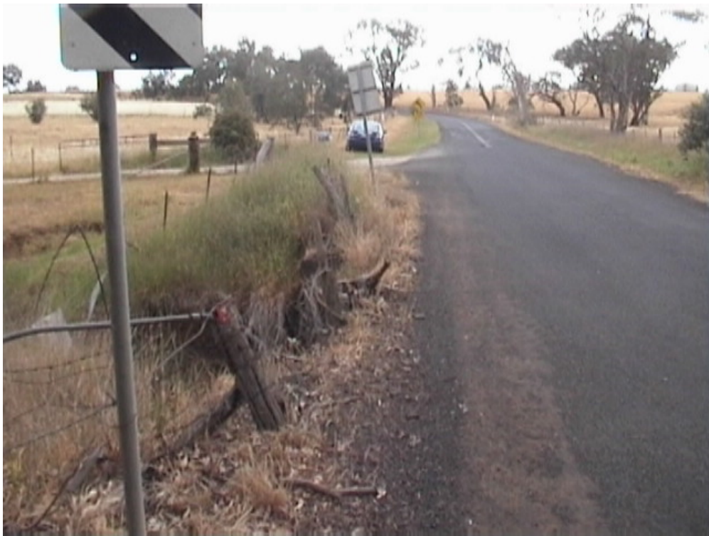
36 – Deficiency Log Item 21
