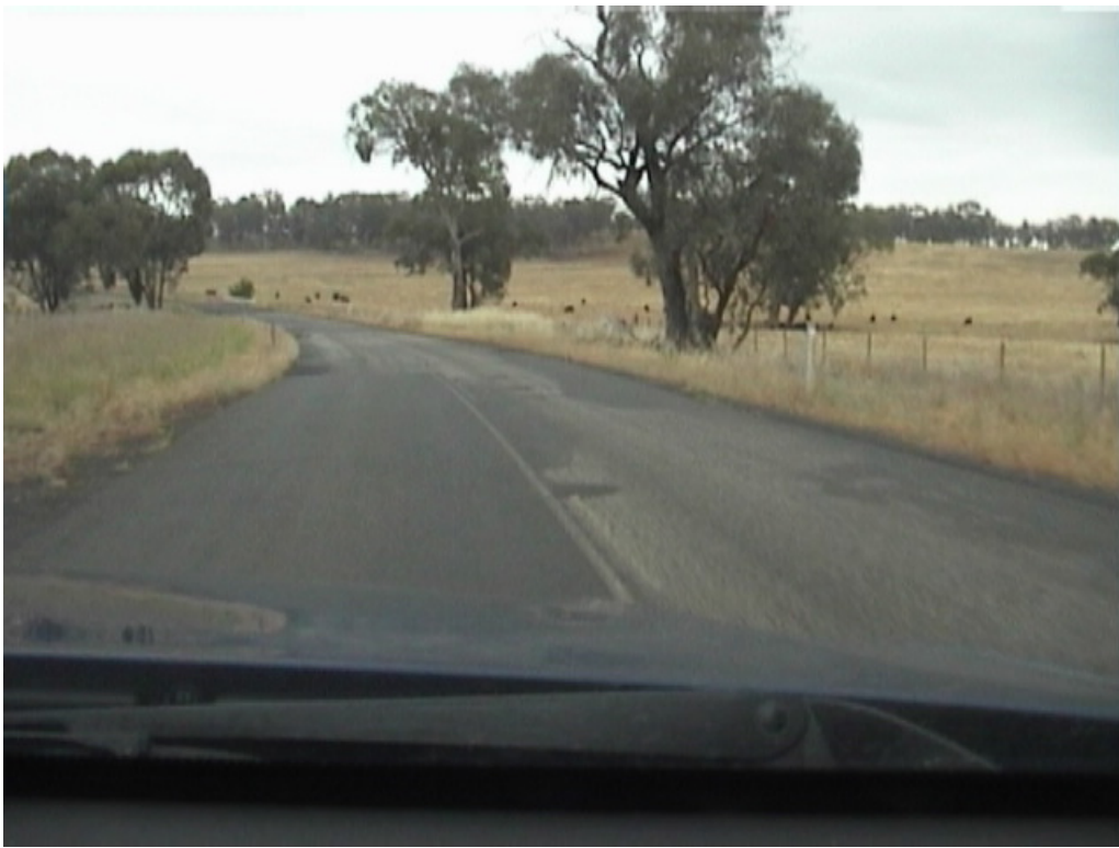
4 - Deficiency Log Item 1
