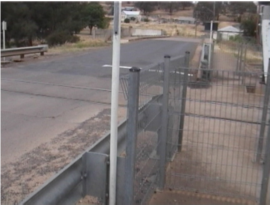
18 – Deficiency Log Item 11
