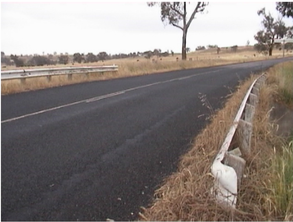
40 - Deficiency Log Item 24
