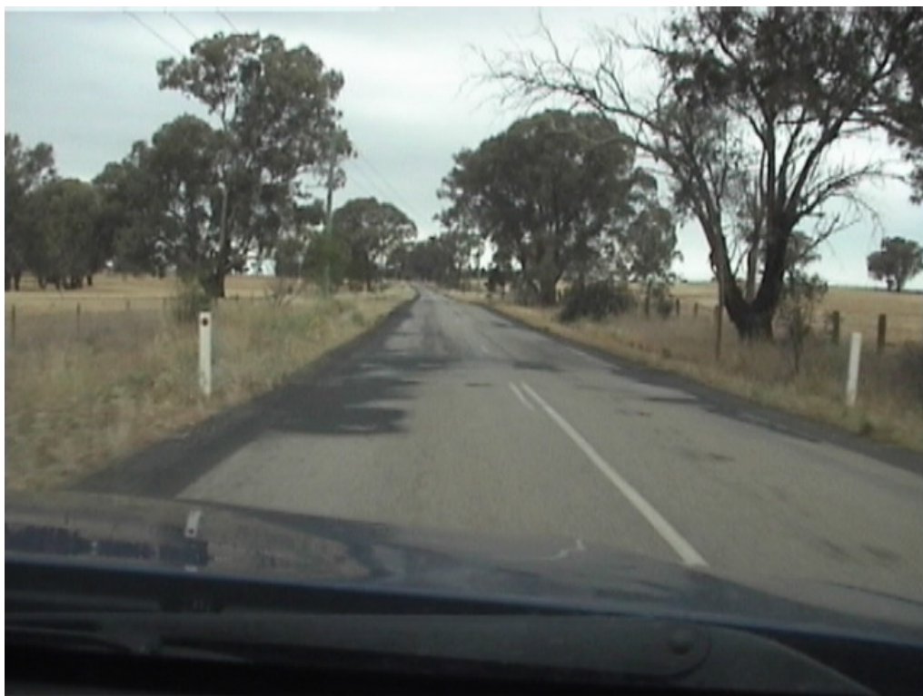
24 – Deficiency Log Item 16
