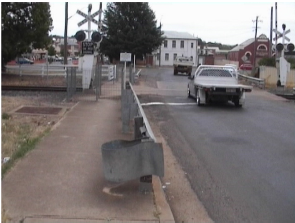
16 – Deficiency Log Item 10
