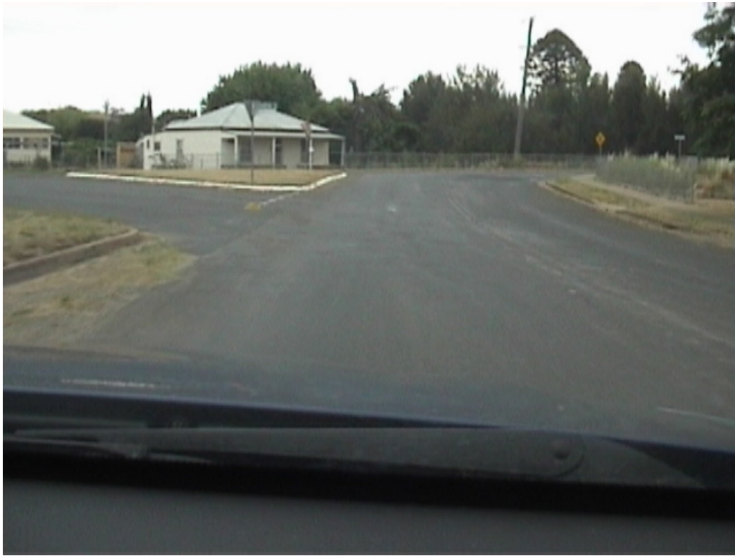
19 – Deficiency Log Item 12 Linemarking at this junction is extremely poor. Given the unusual configuration of the junction, centreline markings are considered imperative for driver appreciation/expectation and operational safety of the junction
