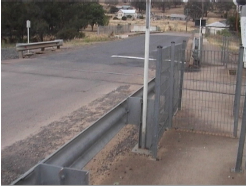
17 – Deficiency Log Item 11 At the Railway Level Crossing there is no provision for disabled wheelchair access. In addition there are no pedestrian controls other than audio (bells) to warn pedestrians of an approaching train.
