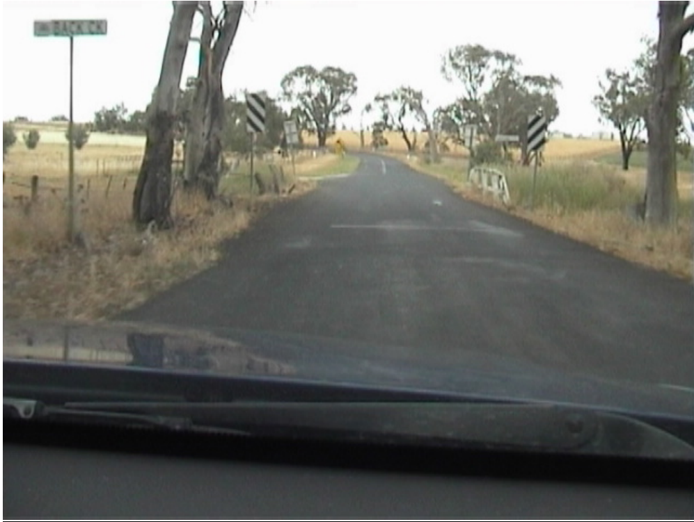
35 – Deficiency Log Item 21
