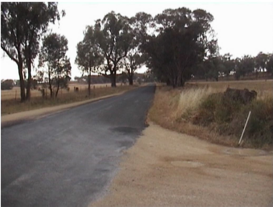
38 – Deficiency Log Item 23
