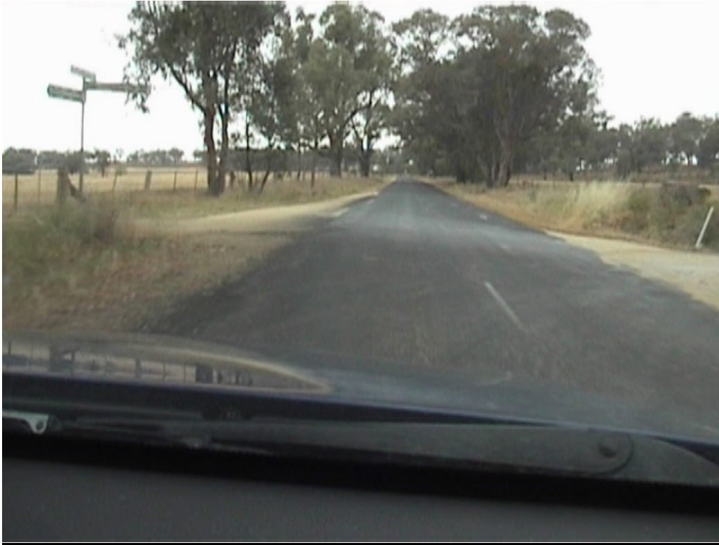
37 – Deficiency Log Item 23 Shades Creek Road services a number of properties and connects through to the Mitchell Highway in the west. At this point the Euchareena Road pavement narrows and tracking of large stones occurs onto the bitumen pavement. It is considered there is a reasonable probability that windscreen damage to vehicles could occur at this location.
