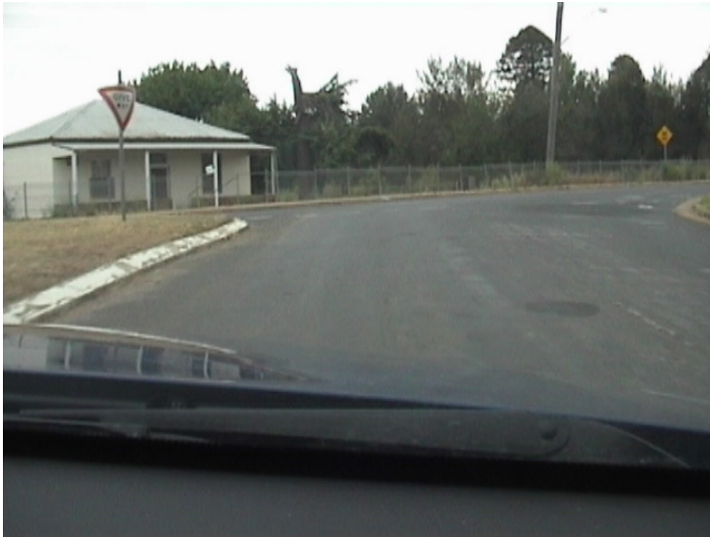
21 – Deficiency Log Item 13 In the south bound direction in Euchareena Road the “Give Way” sign has been damaged and is not perpendicular to oncoming traffic.
