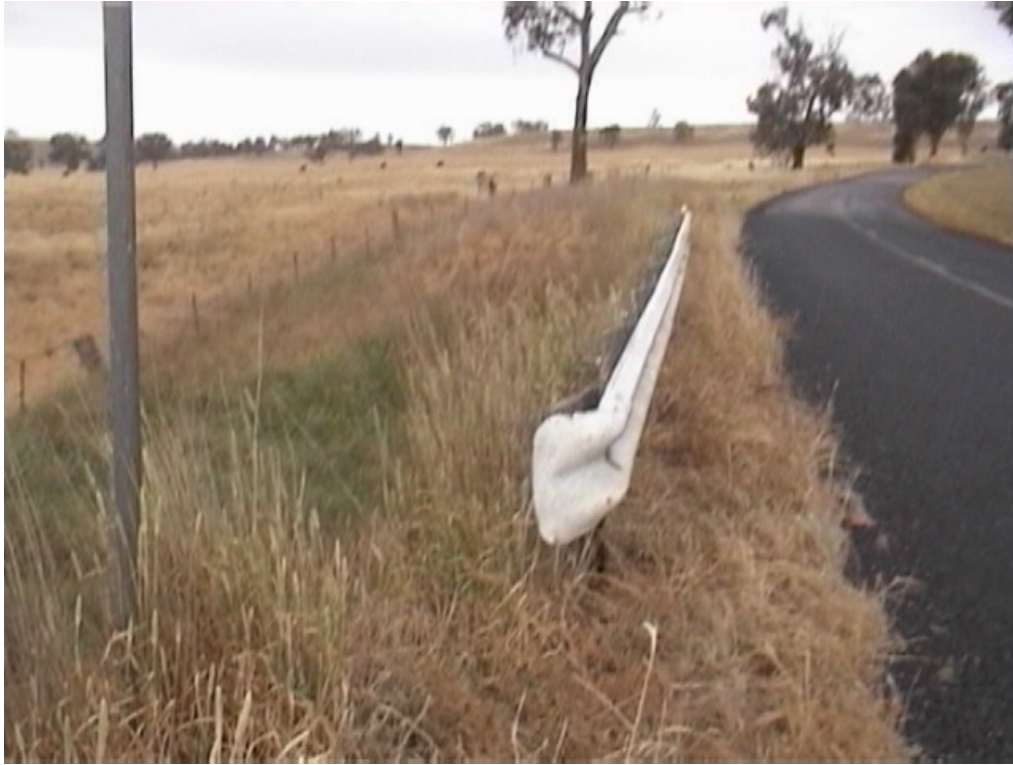
39 - Deficiency Log Item 24 The culvert at Shades Creek accommodates redundant guardrail treatment. The rail is supported by timber posts for its length (deteriorated by white ant and rot) and redundant “fish tail” end treatment.
