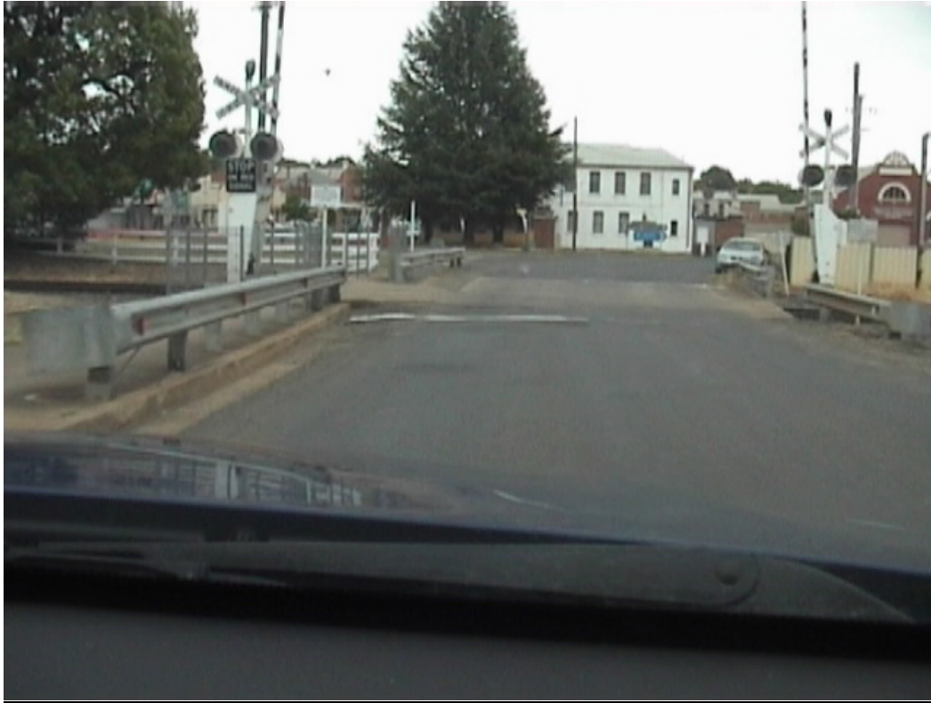
15 – Deficiency Log Item 10 At the Railway Level Crossing the guardrail accommodates redundant Breakaway Cable Terminal (BCT) end treatments. In addition the timber posts supporting the guardrail terminals are rotted and require replacement. The guardrail in the south eastern corner is damaged and requires replacement.
