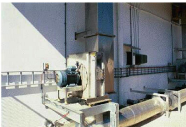
Photo 6-7 Tunnel composting air supply system
