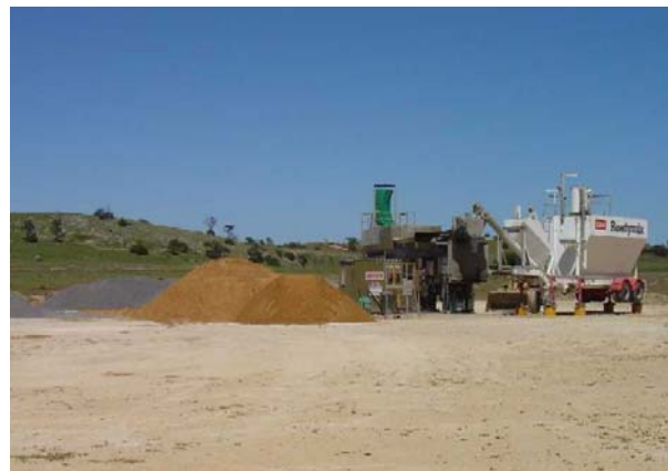
Plate 3.11 – Typical Portable Concrete Batch Plant
