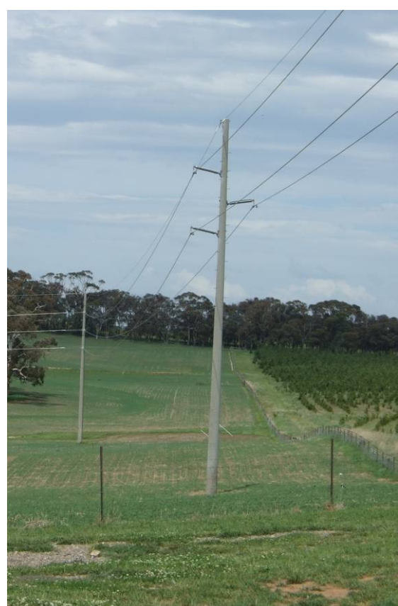
Plate 3.8 – Photo of section of 132 kV line north of Cadia Mine including change in direction
