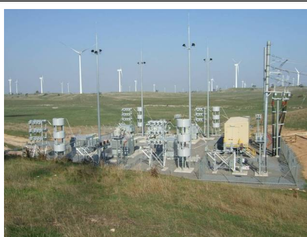
Plate 3.7 – Typical 33 kV switchyard within a secure compound at a South Australian wind farm site
