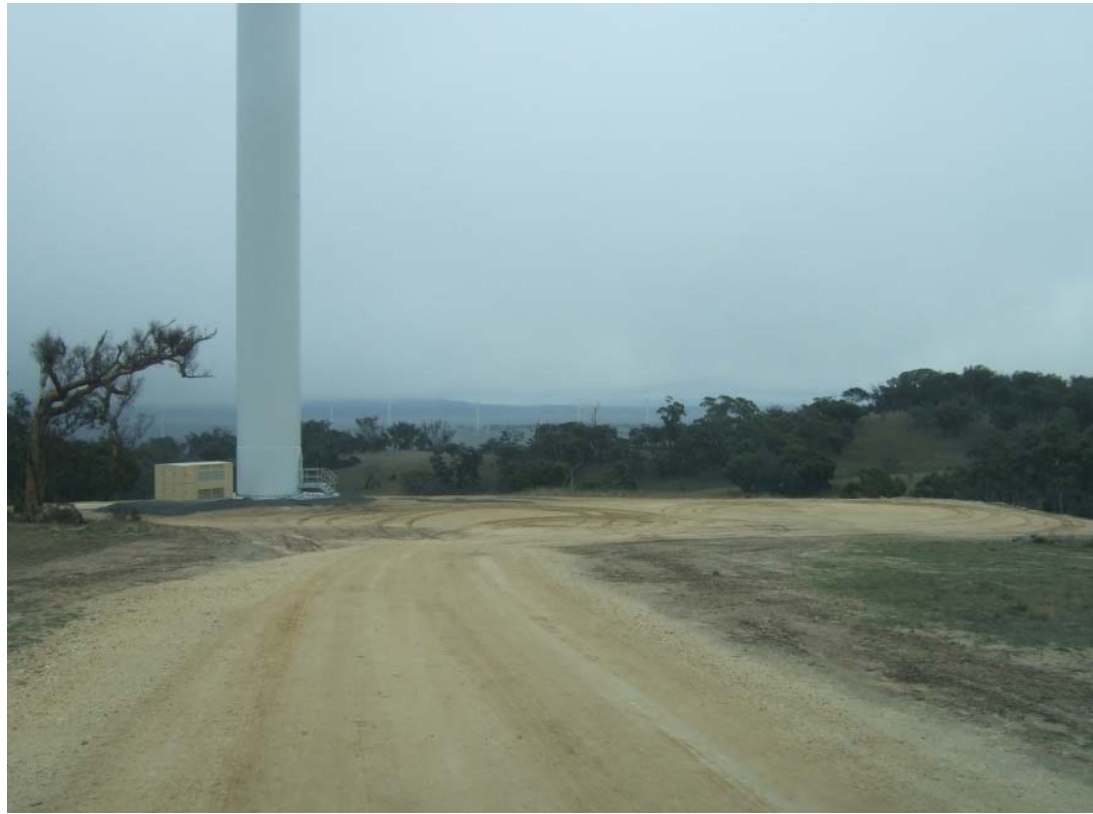
Plate 3.1 – Turbine footing and external padmount 'kiosk' generator transformer adjacent to the hardstand. Depending on the turbine selected, the generator transformer may be located in the nacelle.
