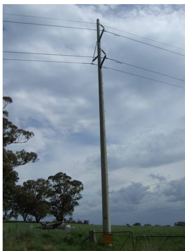
Plate 3.9 – Photo of pole structure for 132 kV line with conductors on alternating sides of pole
