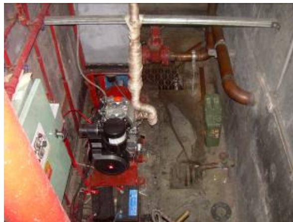
Figure 12 - Basement sprinkler Pump Rooms with tank. Note potential asbestos containing rope around pipe
