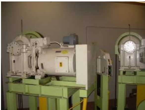
Figure 11 - Motor in Lift Motor Room
