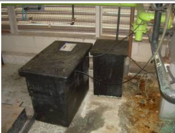
Figure 5 - Cooling tower chemicals in plastic containers
