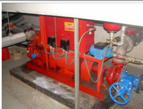
Figure 6 - Rooftop fire hydrant booster pump
