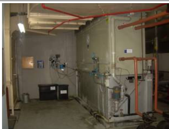
Figure 8 - Location of chemicals for the second cooling tower on the rooftop
