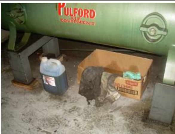
Figure 9 - Air compressor located on rooftop with compressor oil stored beneath
