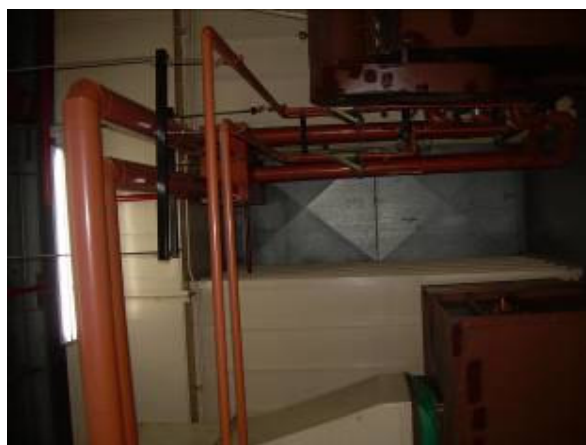
Figure 4 - Cooling tower pipe work, located on the rooftop
