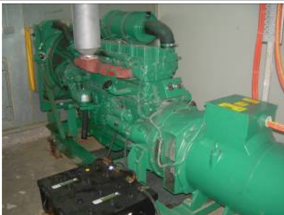
Figure 13 - Diesel backup generator for building, located in the diesel alternator room which is accessed via the car park.
