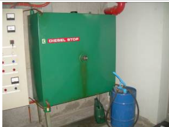
Figure 14 - Diesel up in diesel alternator room. Note drum on floor. Estimated to be approx 100L in capacity
