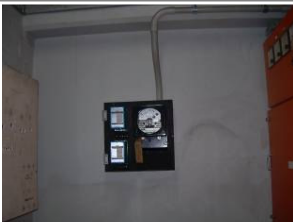
Figure 15 - Potential asbestos containing material in the switchboard room, accessed via Little Spring Street
