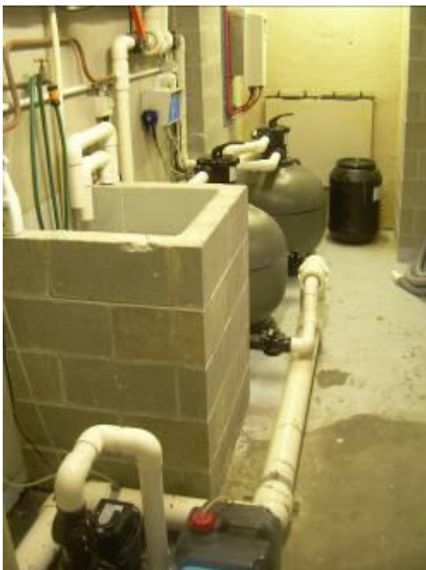
Figure 7 - Pool pump room located on Level 8
