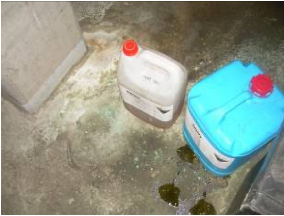
Figure 9 - Chemicals stored in cooling tower plant room on Level 37 of Beau Monde Residential Tower
