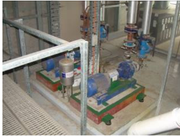
Figure 10 - Plant room on Level 37 containing fire pump systems and hot water systems
