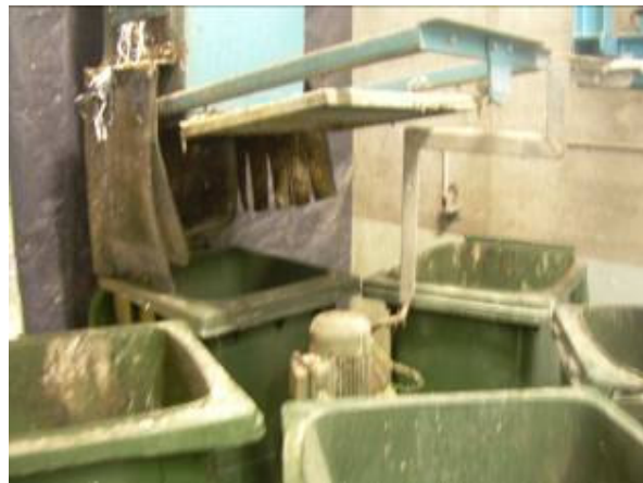
Figure 4 - Waste chute located in the loading dock of Beau Monde Residential Tower
