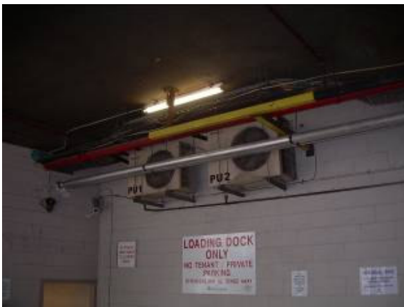
Figure 13 - Air conditioning units located in the loading dock of Berry Square Retail Centre.
