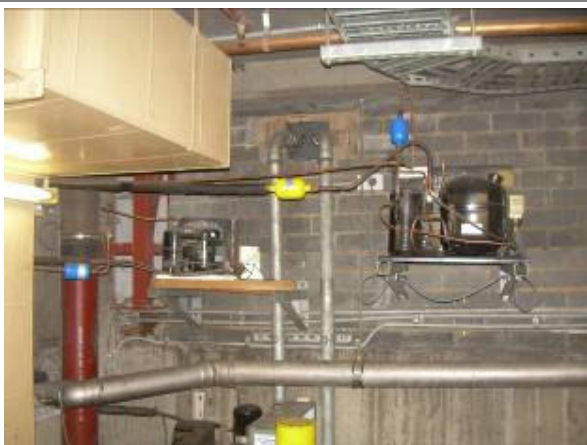
Figure 19 - Small air conditioning units located in Berry Square Car Park
