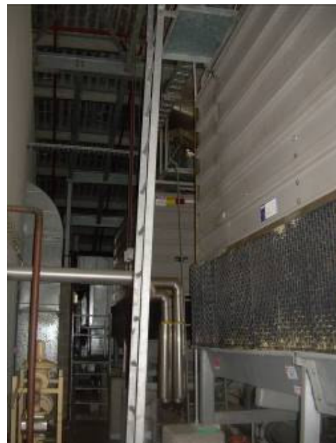
Figure 8 - Cooling tower, located on Level 37 of the Beau Monde Residential Tower.
