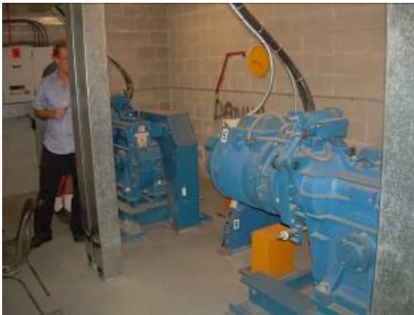
Figure 11 - Lift motor room for Beau Monde Residential Tower.
