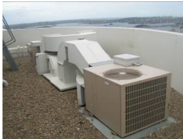
Figure 12 - Air conditioning units on roof of Beau Monde Residential Tower
