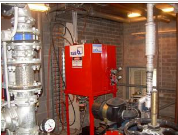
Figure 17 - Fuel tank for the Sprinkler Pump
