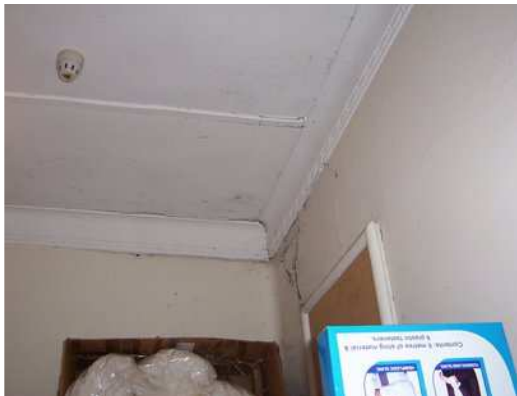
Plate 4.11: Early fibrous plaster ceilings possibly from the 1930's survive in some small rooms
