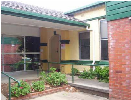
Plate 4.15: View of the original hospital entrance noting the top to the pilasters is plain with no decoration as seen in the photos of the original building.
