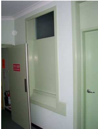
Plate 4.8: An external wall, sill & window now internal due to additions over the years.
