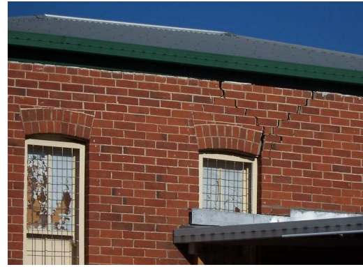
Plate 4.23: The 1916 Operating Theatre building has a number of structural cracks.
