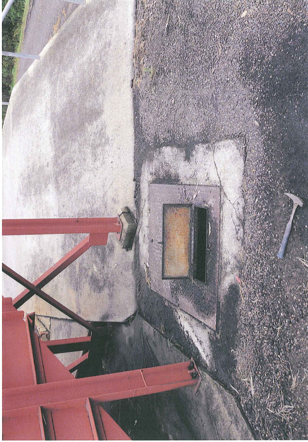
PLATE 4 : A close up view of the underground fuel storage tank with the lid open, next to coal bin.
