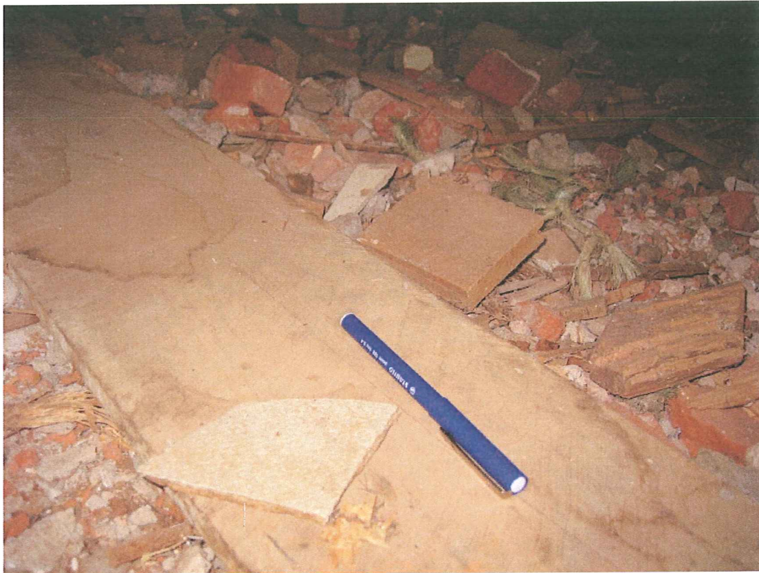
PLATE 6 : Part view of a number of fibrous fragments nixed with demolition debris inside the subfloor of part (physiotherapy) of the main hospital building.
