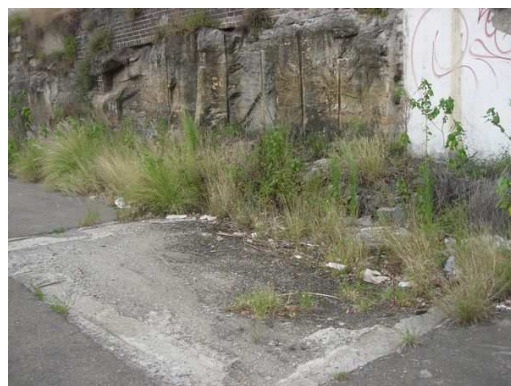
Figure 4.11. Concrete footing of a small shed located in the laneway at the north western corner of the site.
