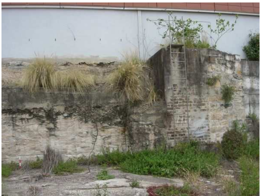
Figure 4.8. The exposed rock face on the western perimeter with sections of brick and sandstone block retaining wall and a raised concrete slab at the base.
