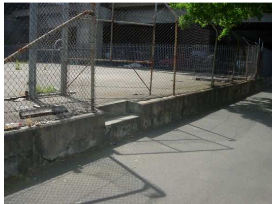
Figure 4.9. The north eastern perimeter of the site stepping down to Pymont Street. This corner of the site is the only part at a higher level than the street.
