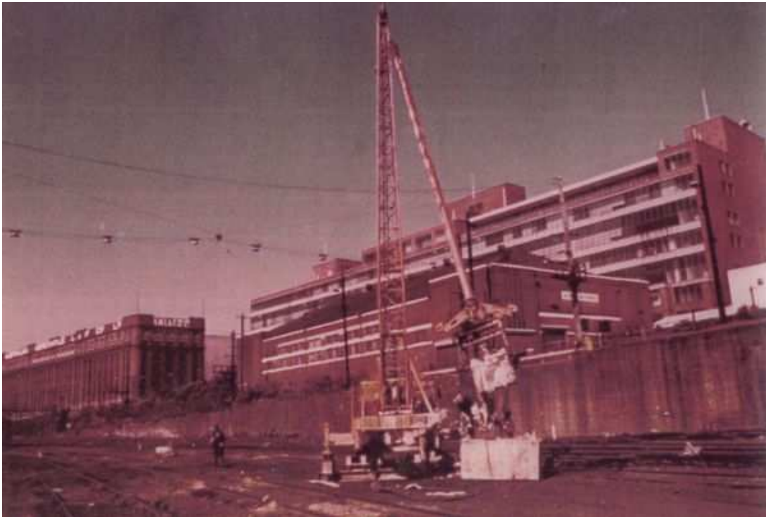
Figure 3.9. 1972 construction of the Murray Street flyover. The Government meat markets building can be seen in the mid ground but the saw tooth buildings have been removed from the site.(Photograph courtesy of SHFA).
