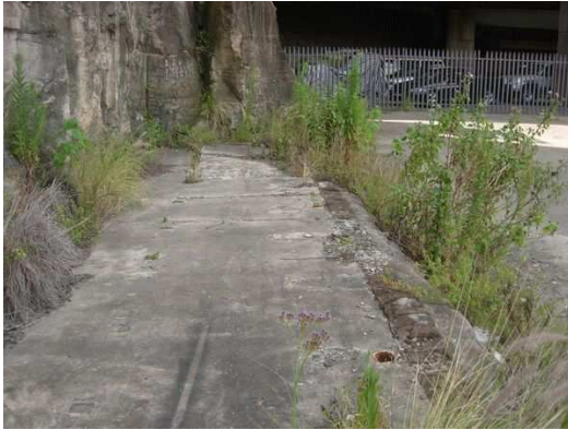
Figure 4.12. Raised concrete slab with evidence of brick walls, toilet cubicles and sewer pipe. This building can be seen built up against the rock face in Figure 3.6.
