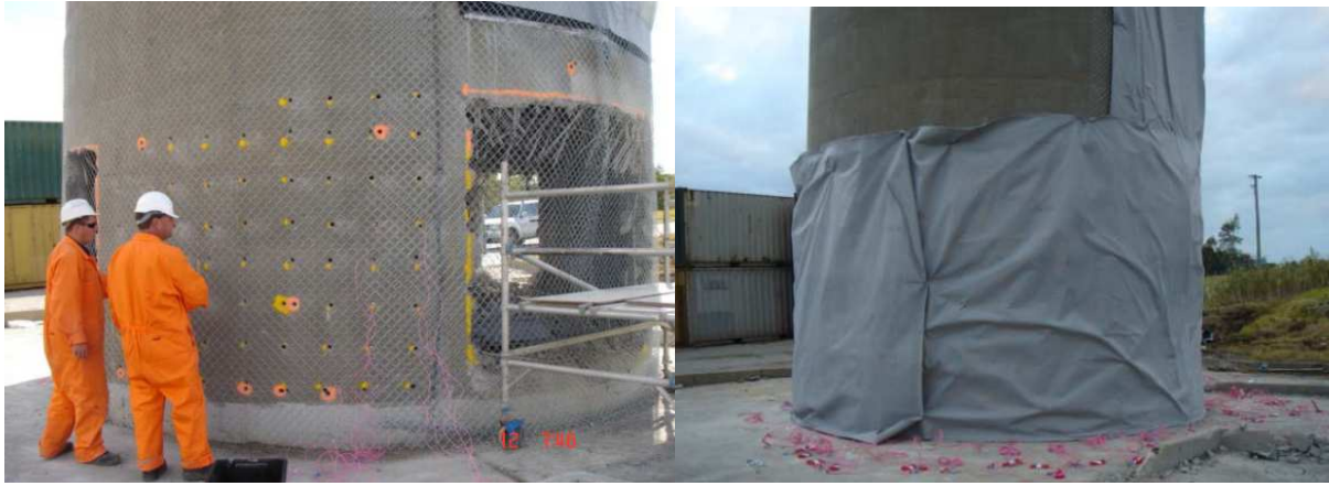
Figure 2: A Chimney Stack Drilled With Blast Holes, Wrapped in Chain Wire and Geo-Fabric
