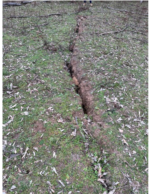
Plate 8: The same crack recorded during Spring 2025
