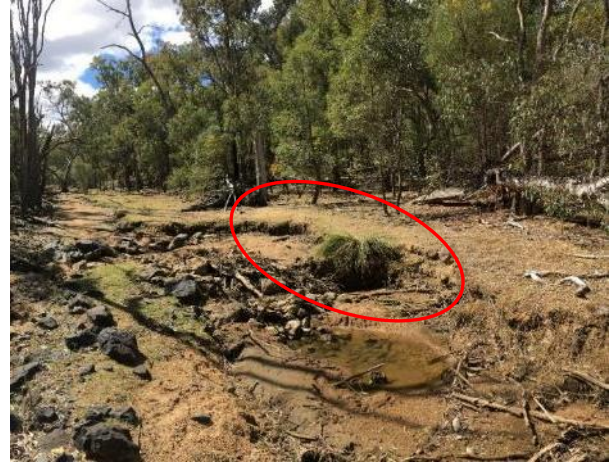
Loss of material evident from LHB in 2017
