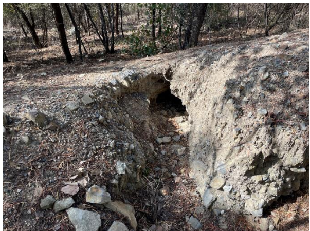
Plate 4: Broken swale resulting in tunnelling in Polygon 9
