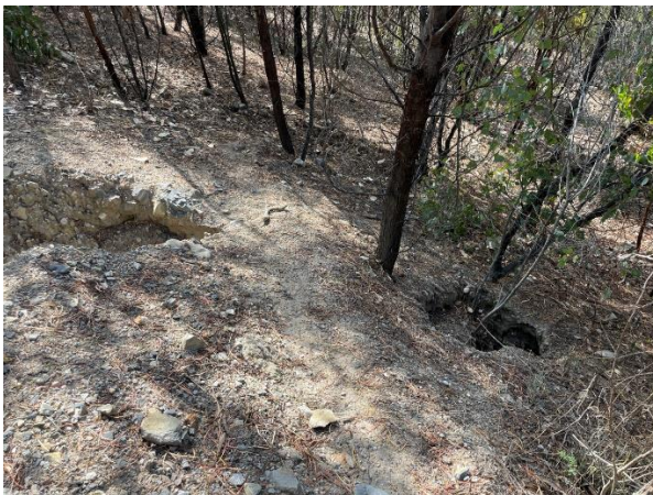
Plate 3: Broken swale resulting in tunnelling in Polygon 9
