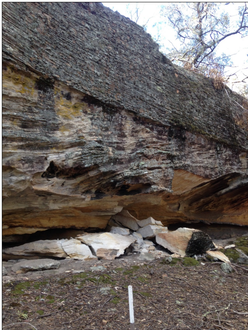
Figure 3a: Rock fall at Aboriginal heritage site Ulan ID# 663 (MC175) above Longwall W4.
