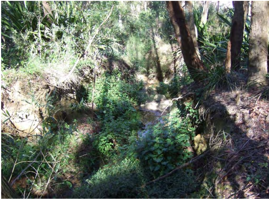
Plate 9: SU4 Creek Bed – view to south west showing eroding creek banks at northern end of creek line
