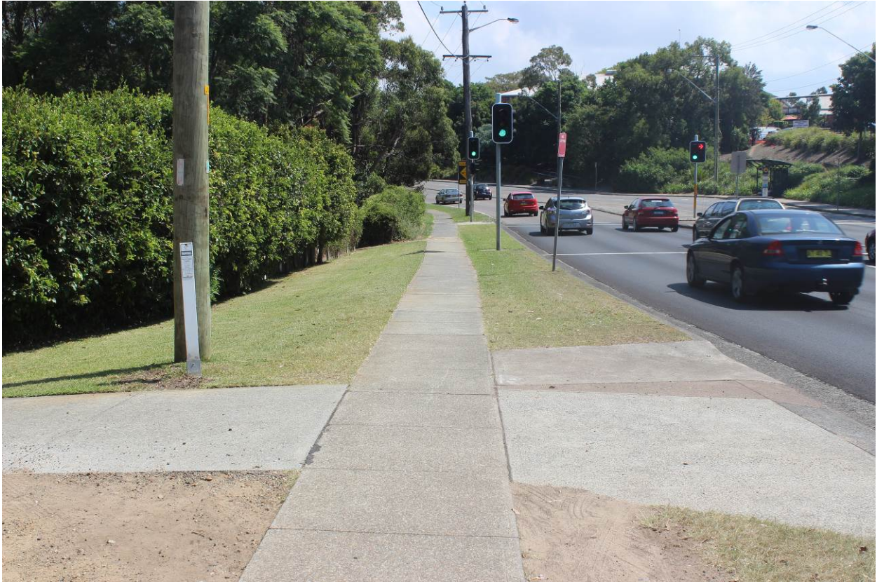
Photograph 7 – Concrete Footpath – Lookout Road
