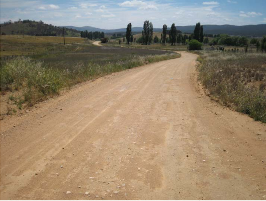
Photo 10: Williamsdale Road unsealed
