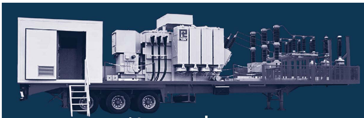
Figure 4 Example of a mobile electrical sub-station.
