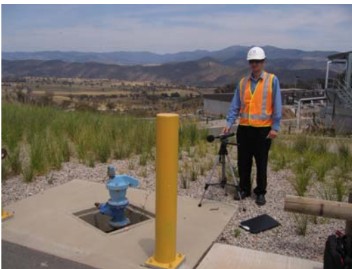
Figure 5 Example photograph of an air valve from a similar pipeline project.
