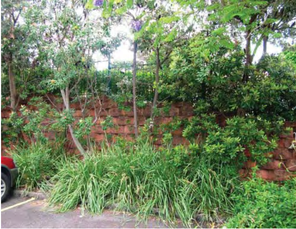
Figure 3.19 The curved concrete block retaining wall of the to the north of the subject site.
