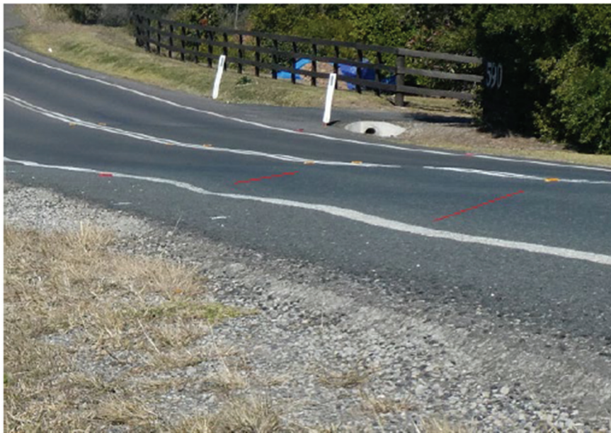
Fig. 6.9 Compression bumps in Menangle Road (Source: Network Solutions)
