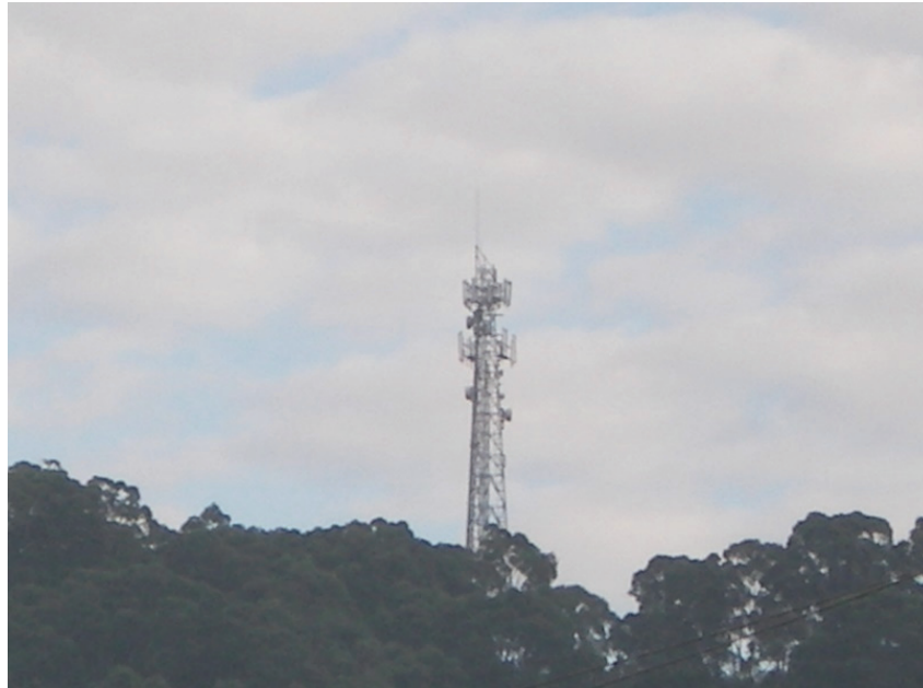
Fig. 6.21 Mobile phone telecommunications tower
