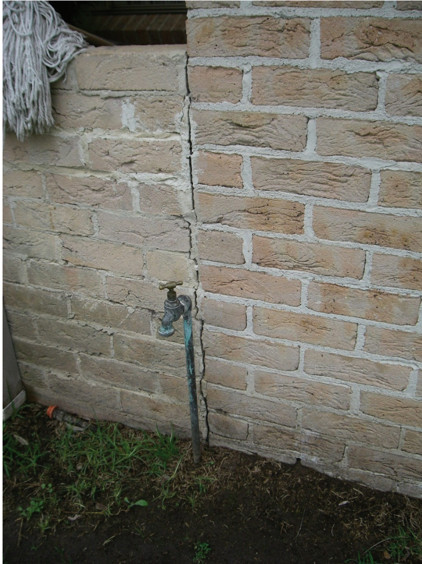
Fig. B.2 Example of crack in mortar only
