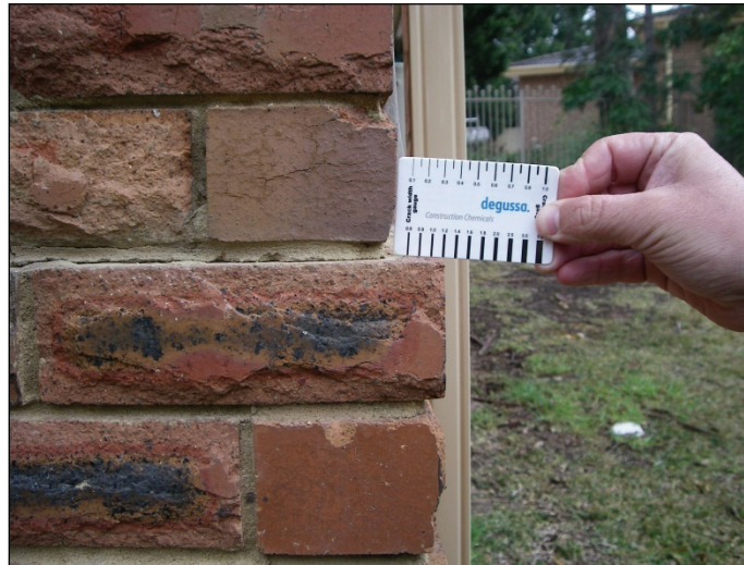
Fig. B.1 Example of slippage on damp proof course
