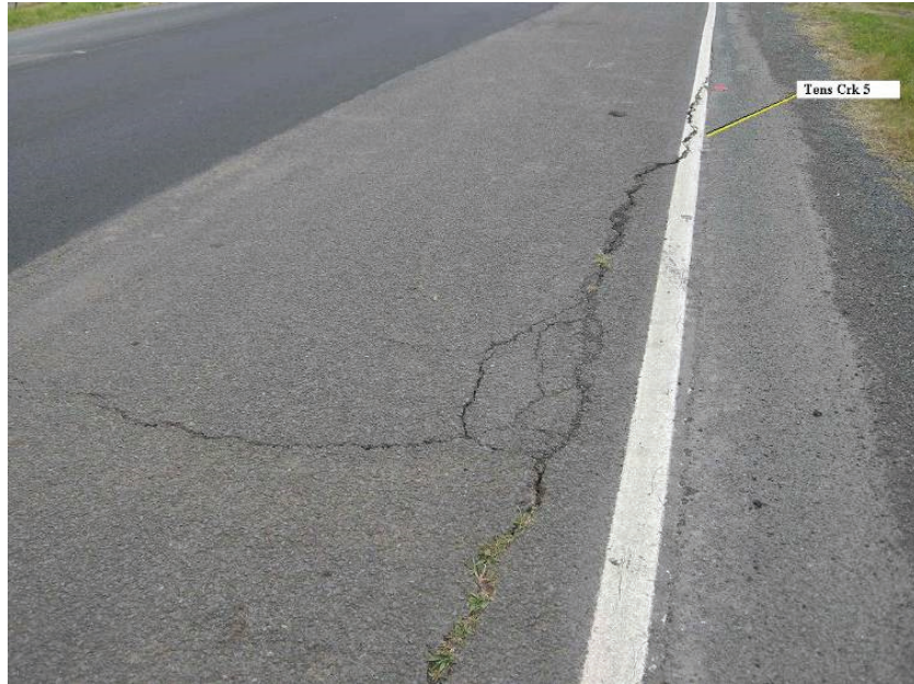
Fig. 6.8 Tension crack in Appin Road above West Cliff Longwall 32 (Source: Colin Dove)
