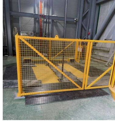
Plate 2: Heavy duty shaft blast doors
