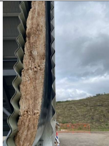
Plate 4: Double skin cladding and noise insulation
