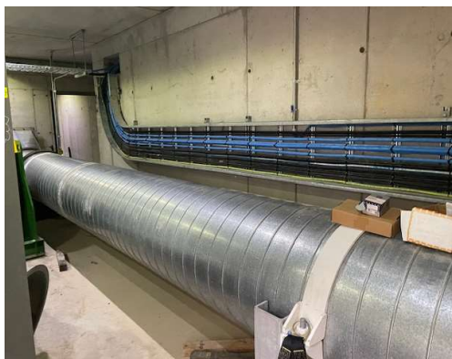
Plate 5: Underground concrete encased shaft ventilation system
