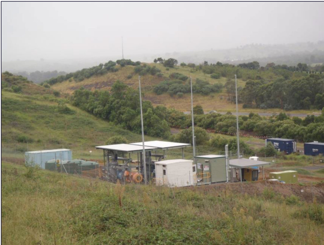
Plate 4: Extraction Plant (Area 7 – now decommissioned)
